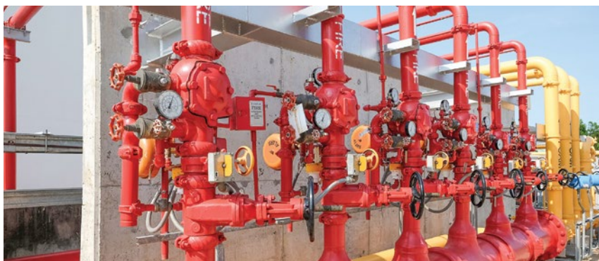
Engineered piping and valves form the backbone of any foam-based fire protection system and require careful calibration and maintenance to support the shift to fluorine-free agents.
